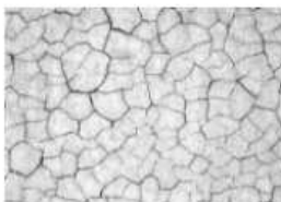
a) Mud Cracking
