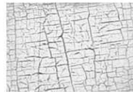
c) Age Cracking
